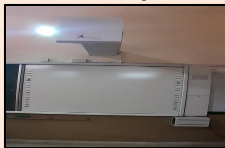
THE BRIO'S SMART BOARD INSTALLED IN MAIN BLOCK MATHS LAB
